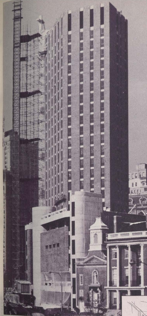
Building as it appeared January 2, 1968. Temporary elevator staging at front of structure and contractor's hoisting engine on sidewalk have since been removed.
