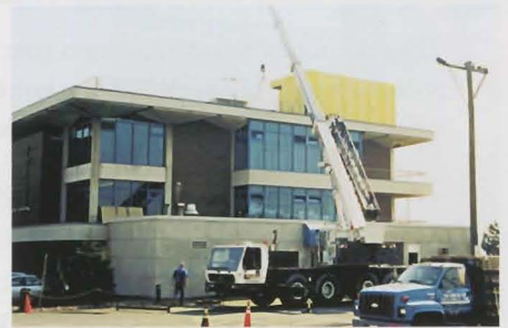
A work crew replaced all of the windows and placed new heating and air conditioning units on the roof as renovations continue at the International Seafarers' Center.
