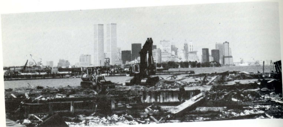
View of the harbor clearing area, shows construction crews demolishing old piers.
